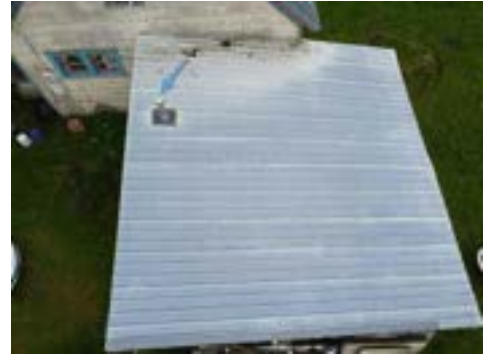
Vent Stack Cap Damaged - Flat Roof Structure
