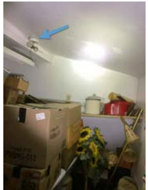
Light Fixture Cover Missing - Garage
