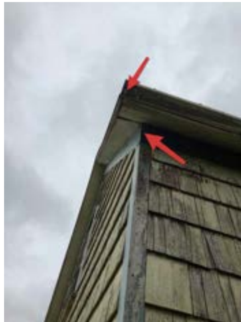
Fascia/Eave Wood Rot (Representative Picture)
