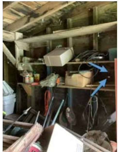
Wall Penetrations - Garage (Representative Picture)
