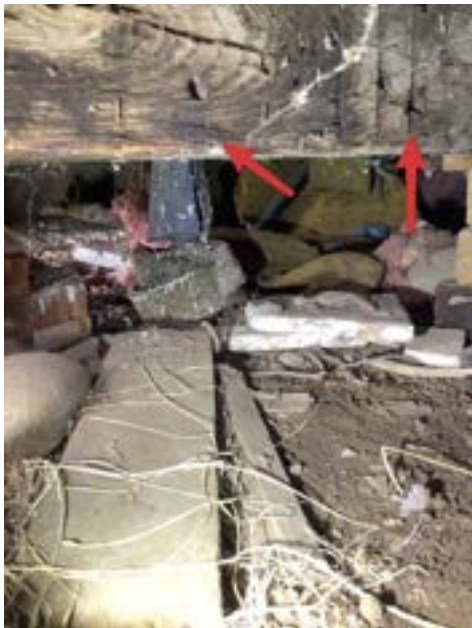
Sub-Floor Structure Wood Rot/Damage - Crawl Space (Representative Picture)
