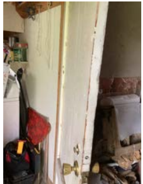
Door Does Not Meet Separation Requirements - Garage
