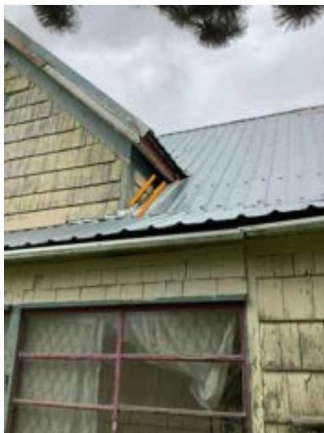
Siding in Contact With Roof (Representative Picture)
