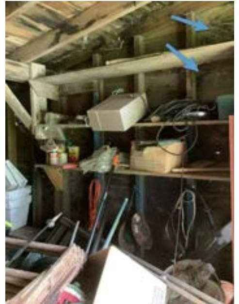
Wall Surface Staining/Discoloration - Garage (Representative Picture)
