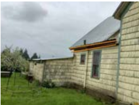
Gutter System Damaged/Not Present (Representative Picture)
