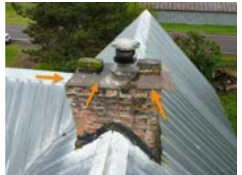
Corroded Chimney Crown - Center Ridgeline
