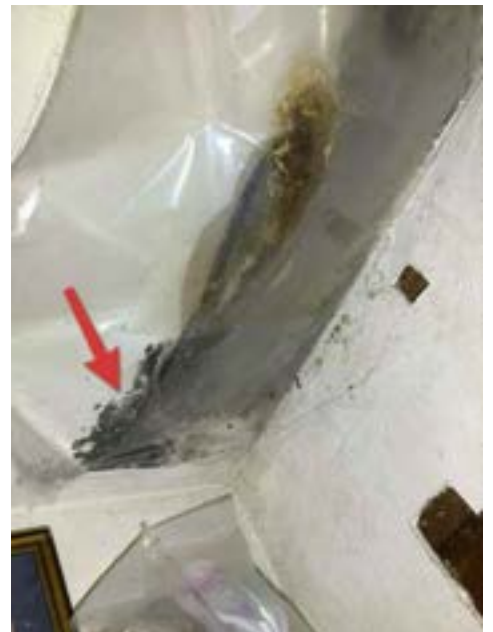
Signs of Possible Microbial Growth - Bedroom (First Floor - On Right)
