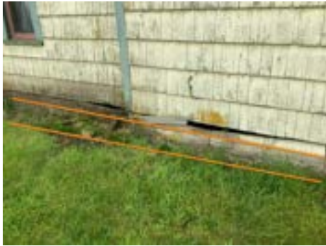
Skirting in Contact With the Ground (Representative Picture)
