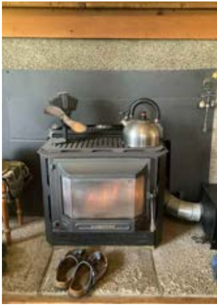
Gas Fireplace - Living Room (First Floor)
