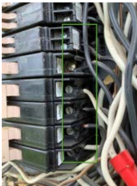
15 & 20 amp Breakers - Main Electrical Panel (Side B)
