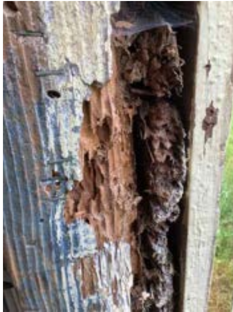
Signs of Wood Destroying Insects (Representative Picture)
