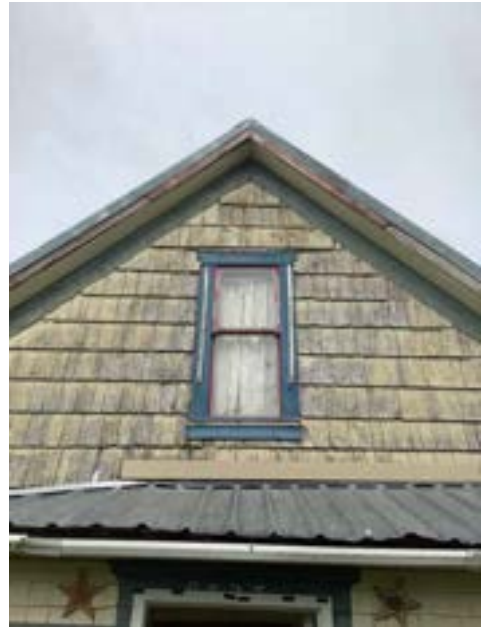
Siding/Trim Paint Deteriorating (Representative Picture)
