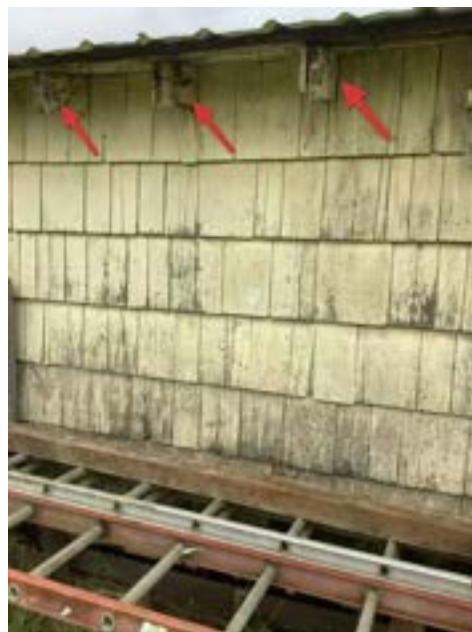
Rafters Wood Rot (Representative Picture)
