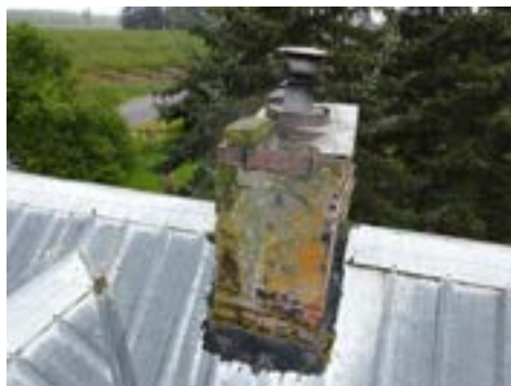
Moss Growth on Chimney Structure - Center Ridgeline (Representative Picture)
