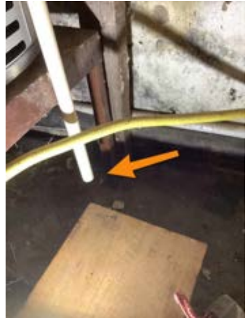
TPR Valve Discharges Onto Floor - Utility Room (First Floor)
