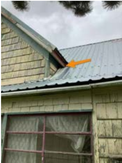
Fascia in Contact With the Roof (Representative Picture)
