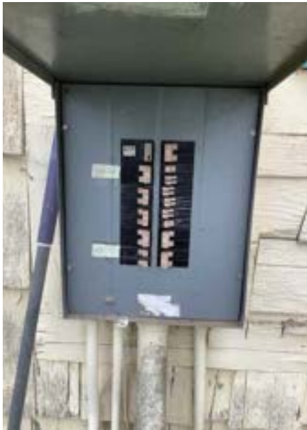
Main Electrical Panel - Cutler Hammer (Side B)
