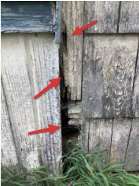
Siding/Trim Wood Rot (Representative Picture)
