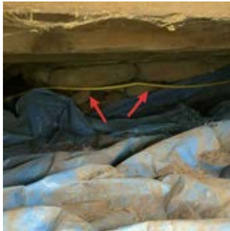
Floor Structure Improperly Braced - Crawl Space (Representative Picture)
