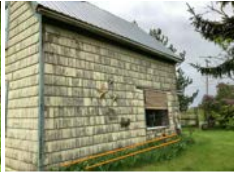
Skirting in Contact With the Ground (Representative Picture)
