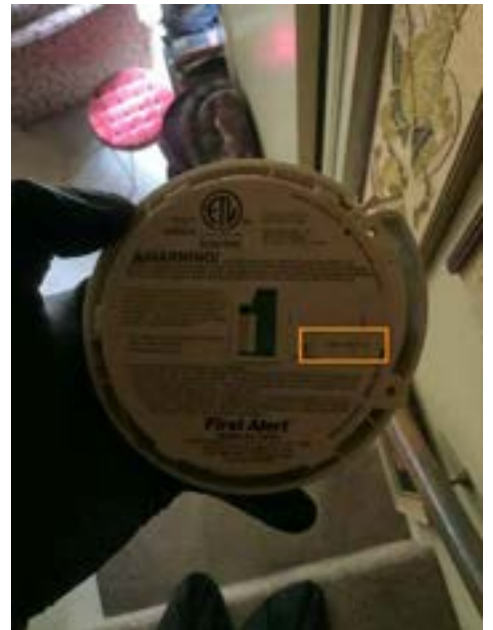
Smoke Detector Exceeds Age Requirements - Stairway (First Floor to Second Floor) (Dated 2012)
