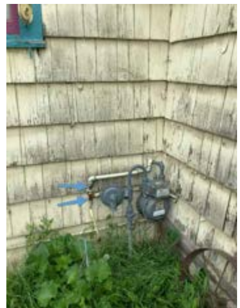
Corroded Gas Supply Line - Side B
