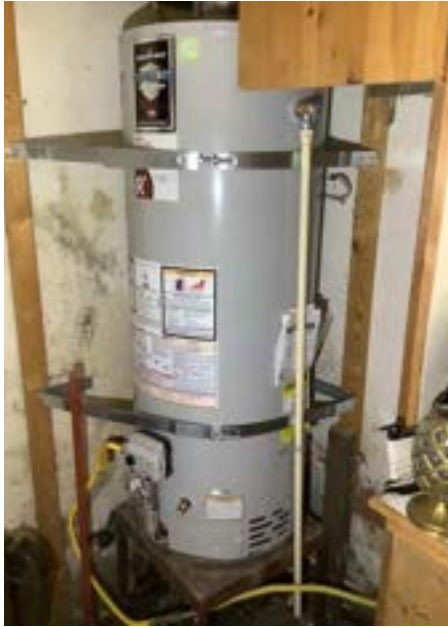
Water Heater - Bradford & White (First Floor - Utility Room)
