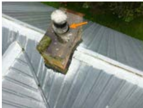
Gap Around Vent Stack - Center Ridgeline
