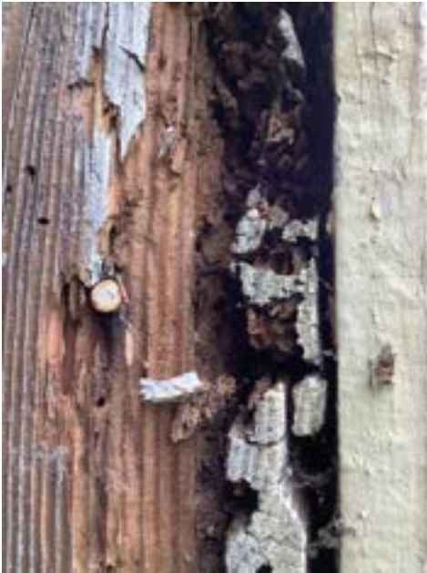
Signs of Wood Destroying Insects (Representative Picture)
