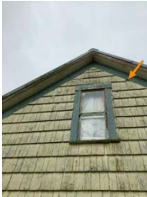
Section(s) of Missing Siding (Representative Picture)
