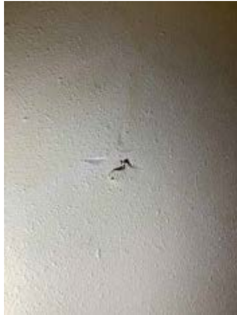
Wall Surface Damage (Representative Picture)
