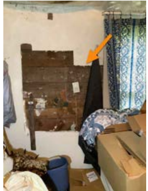
Section of Drywall Missing - Bedroom (First Floor - On Right)
