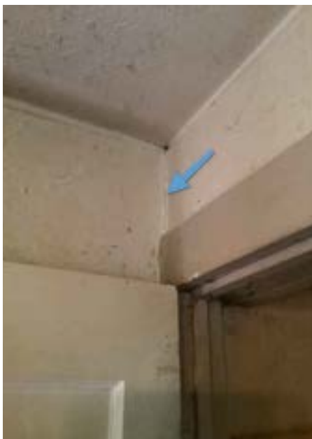
Wall Surface Crack(s) (Representative Picture)
