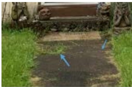
Walkway Crack(s) - Side A (Representative Picture)
