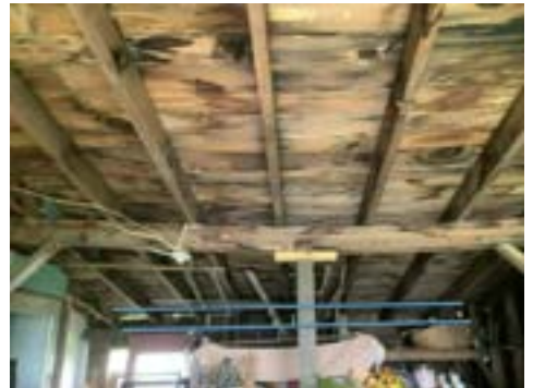
Ceiling Structure Gaps - Garage (Representative Picture)
