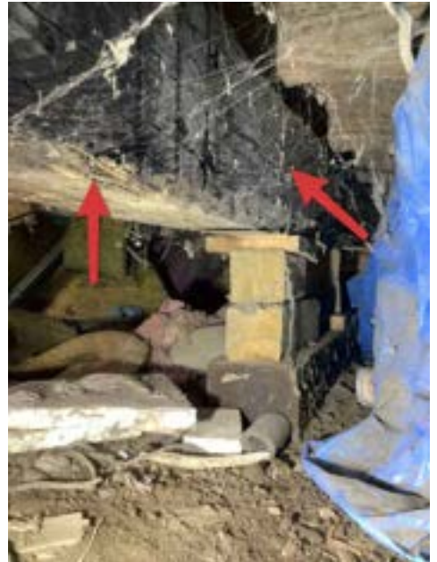
Sub-Floor Structure Wood Rot/Damage - Crawl Space (Representative Picture)
