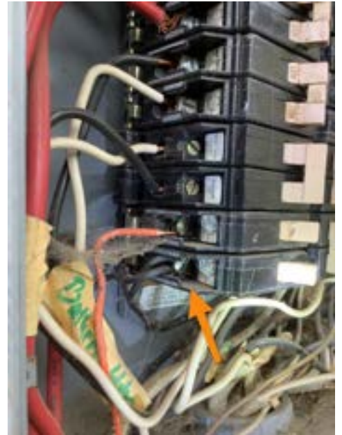
Breaker #23 Incorrectly Wired - Side B
