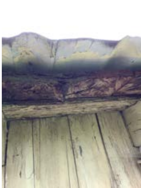
Roof Decking Wood Rot (Representative Picture)
