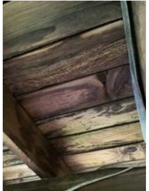
Signs of Wood Destroying Insects (Representative Picture)
