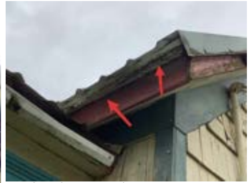
Roof Decking Wood Rot (Representative Picture)
