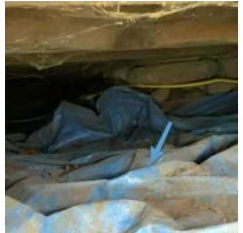
Incorrect Type of Vapor Barrier Material - Crawl Space (Representative Picture)
