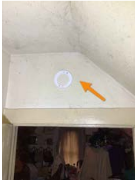
Smoke Detector(s) Not Present - Second Floor (Representative Picture)
