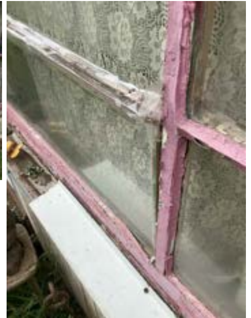
Window Trim/Frame Wood Rot (Representative Picture)
