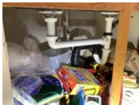
No Garbage Disposal System Present - Kitchen (First Floor)
