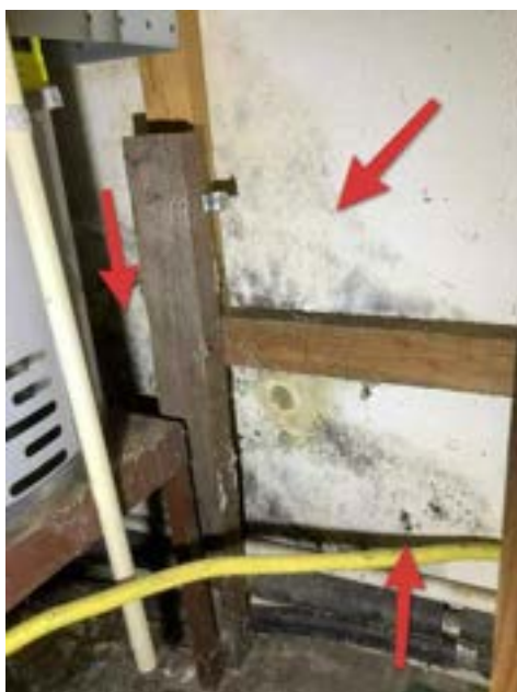
Signs of Possible Microbial Growth - Utility Room (First Floor)
