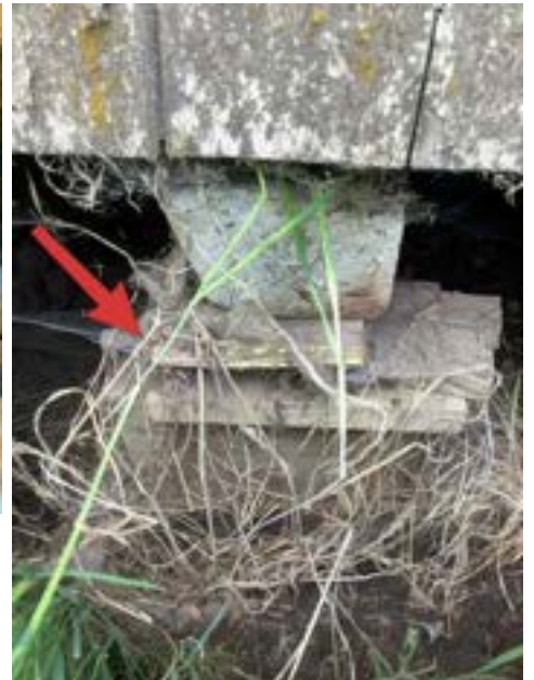
Floor Structure Improperly Braced - Crawl Space (Representative Picture)
