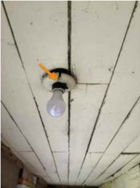
Light Fixture Damaged - Side A
