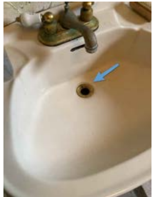
Drain Stop Missing - Full Bathroom (First Floor)
