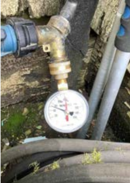
Water Pressure Readings Observed Between 55 & 60 PSI
