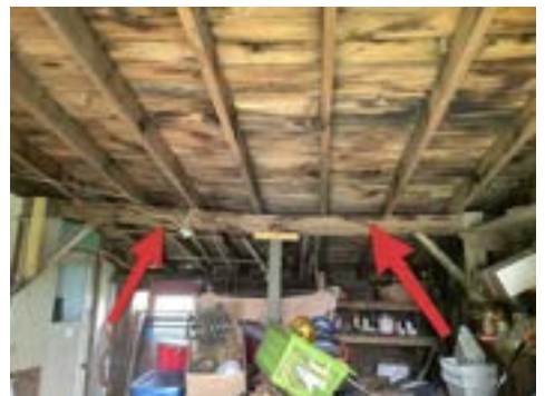
Ceiling Structure Sagging - Garage
