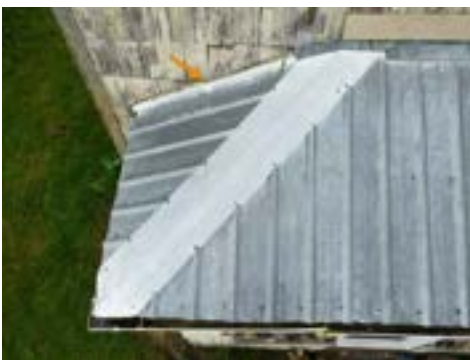
Siding in Contact With Roof (Representative Picture)
