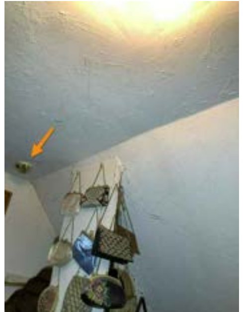
Smoke Detector(s) Damaged (Representative Picture)
