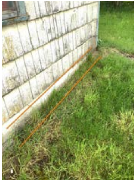
Skirting in Contact With the Ground (Representative Picture)
