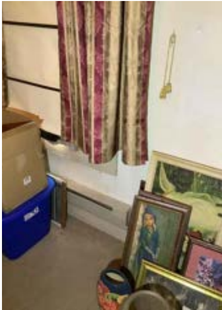
Electric Baseboard Heater(s) (Representative Picture)
