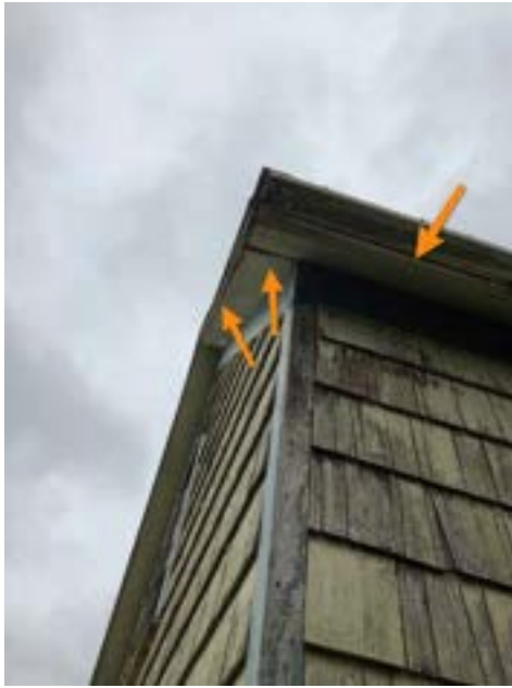
Picture 1a - Eave Panel Gaps (Representative Picture)
