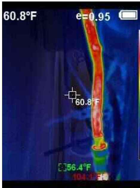
Thermal Image - Half Bathroom Sink (First Floor)
