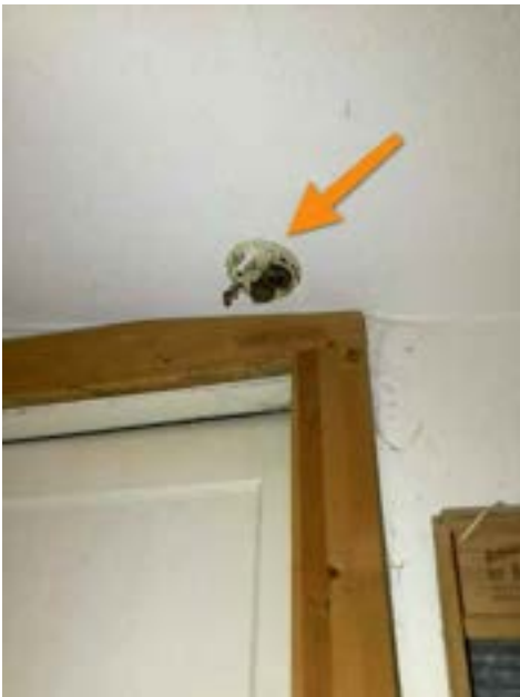
Smoke Detector(s) Damaged (Representative Picture)
