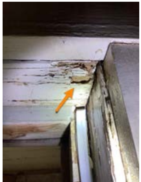
Signs of Wood Destroying Insects (Representative Picture)
