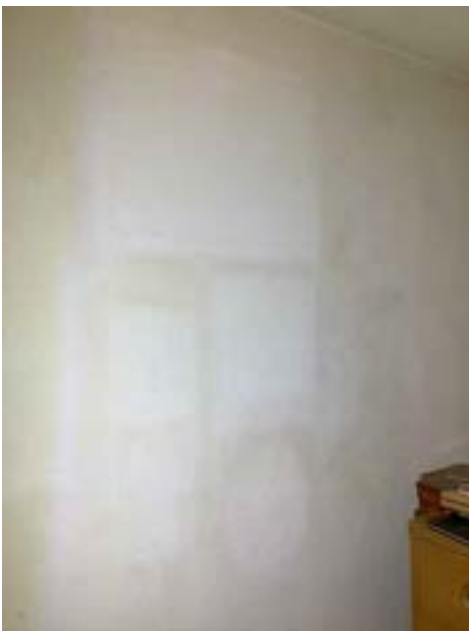
Staining/Discoloration on Wall Surface(s) (Representative Picture)
