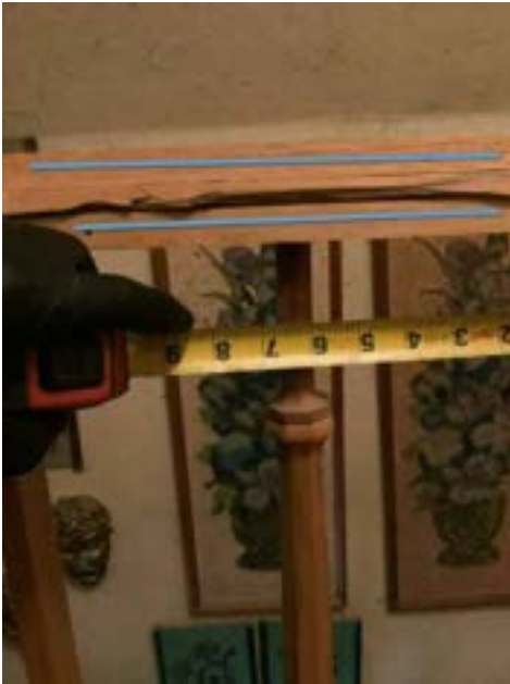
Guardrail Damaged - Hallway (Second Floor)
