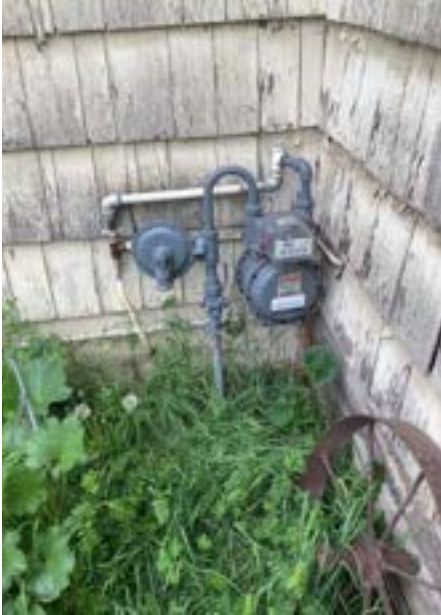
Gas Meter - Side B
