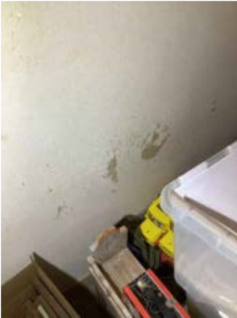
Wall Surface Damage (Representative Picture)
