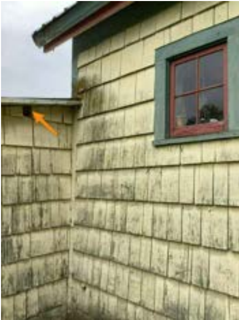
Section(s) of Missing Siding (Representative Picture)
