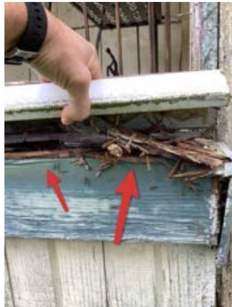
Siding/Trim Wood Rot (Representative Picture)
