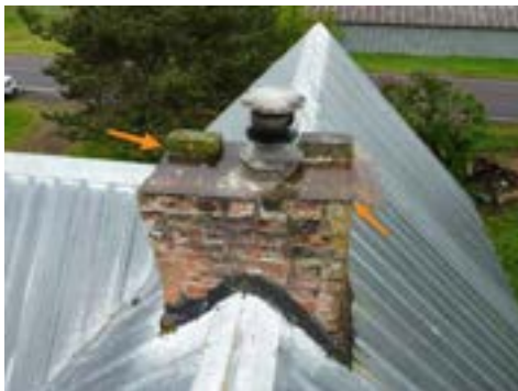
Chimney Crown Not Properly Installed - Center Ridgeline
