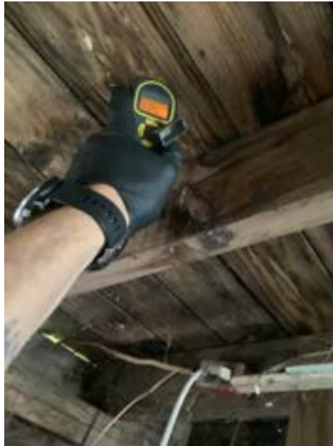
Ceiling Structure Wood Rot - Garage (Representative Picture)
