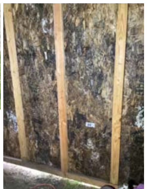
Garage Door Wood Rot - Side B (Representative Picture)
