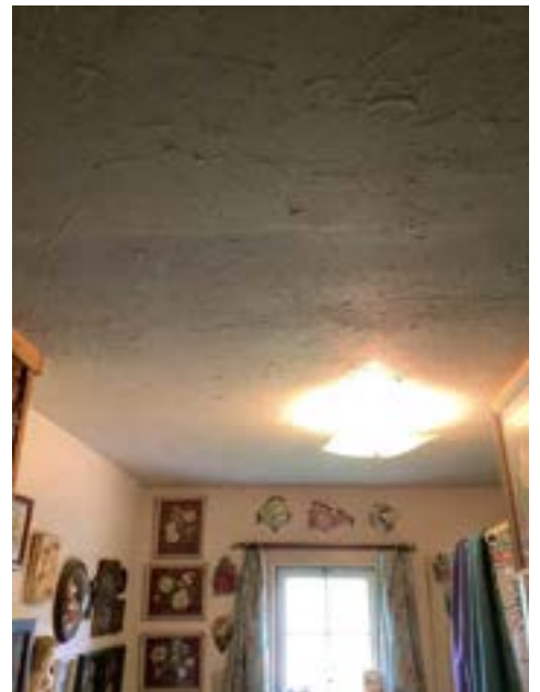
Exhaust System Not Present - Full Bathroom (First Floor)
