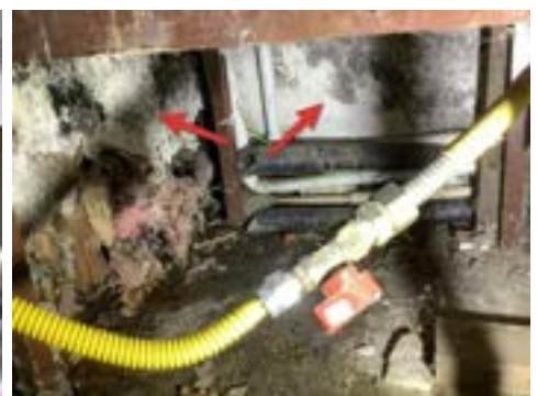
Signs of Possible Microbial Growth - Utility Room (First Floor)
