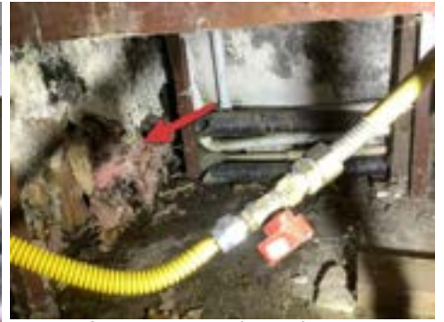
Signs of an Active Leak - Utility Room (First Floor)
