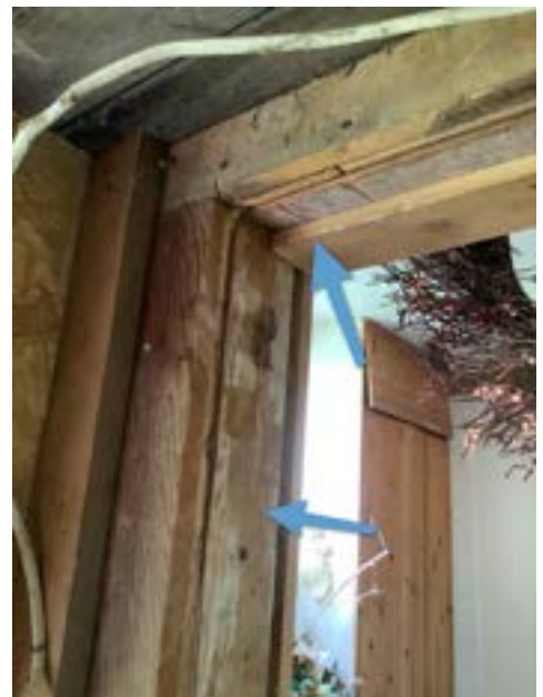
Weather-Stripping Not Present - Garage
