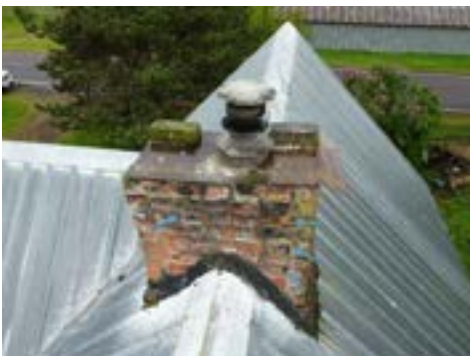
Chimney Mortar Deteriorating - Center Ridgeline
