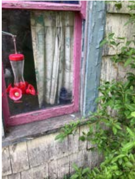
Siding/Trim Paint Deteriorating (Representative Picture)
