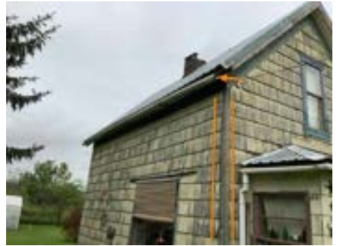
Gutter System Damaged/Not Present (Representative Picture)
