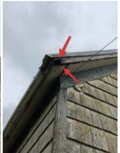
Fascia/Eave Wood Rot (Representative Picture)
