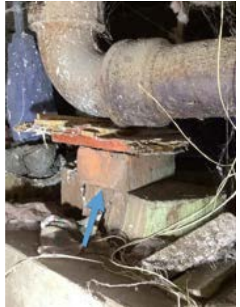
Improperly Supported Drain/Waste Piping - Crawl Space
