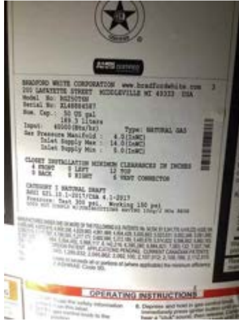
Water Heater - Bradford & White Manufacturer Label (First Floor - Utility Room)
