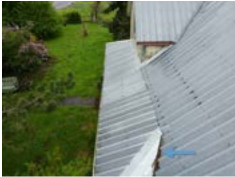
Corroded Roof Covering (Representative Picture)
