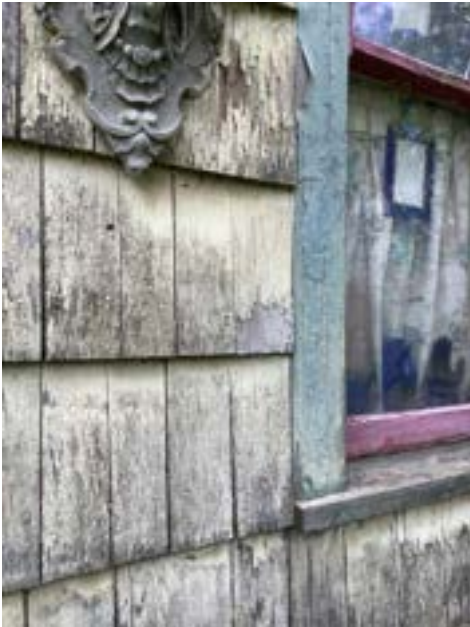
Siding/Trim Paint Deteriorating (Representative Picture)
