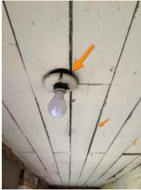
Picture 1b - Eave Panel Gaps (Representative Picture)
