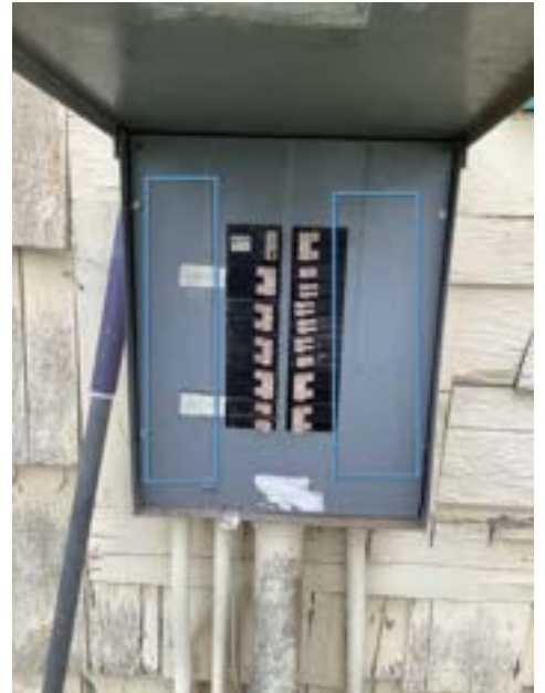
Insufficient Labeling of Electrical Panel - Side B
