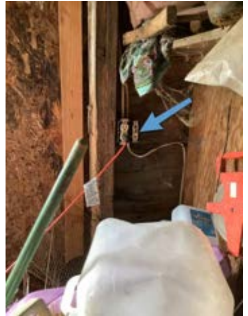
Outlet Cover Plate Missing - Garage
