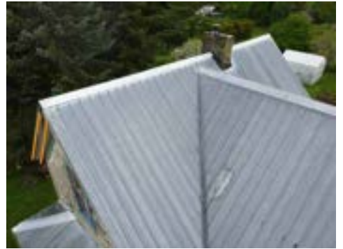
Picture 2 - Fascia/Eave Gap(s) (Representative Picture)
