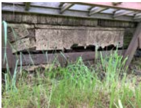
Skirting Wood Rot (Representative Picture)
