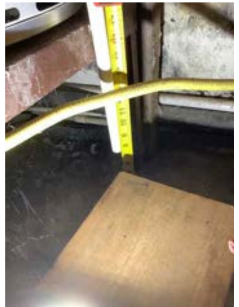
Incorrect Length of TPR Valve Piping - Utility Room (First Floor)
