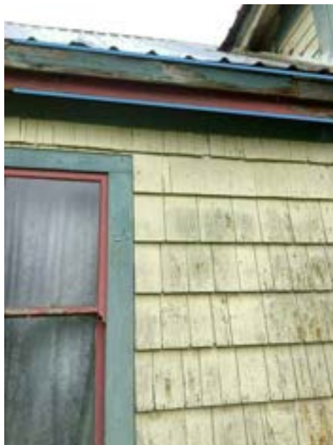
Fascia/Eave Paint Deteriorating (Representative Picture)
