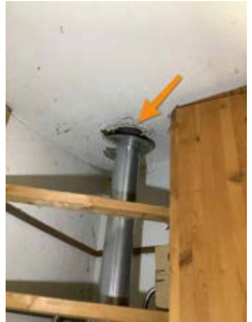
Ceiling Damaged - Utility Room (First Floor)
