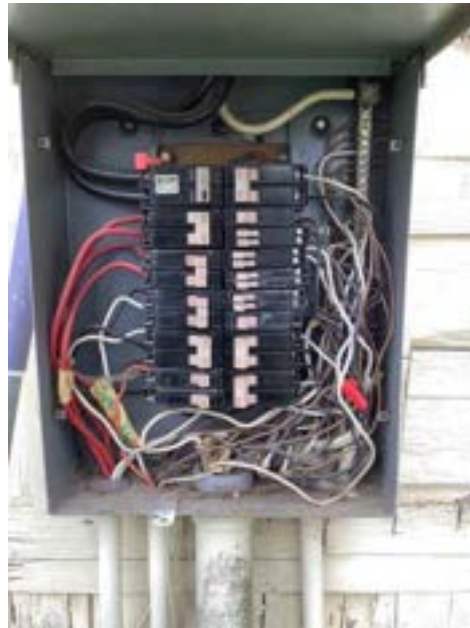
Main Electrical Panel - Cover Removed (Side B)
