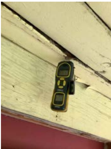
Fascia/Eave Wood Rot (Representative Picture)
