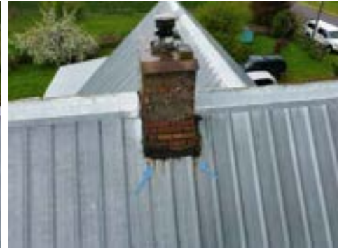
Corroded Roof Covering (Representative Picture)
