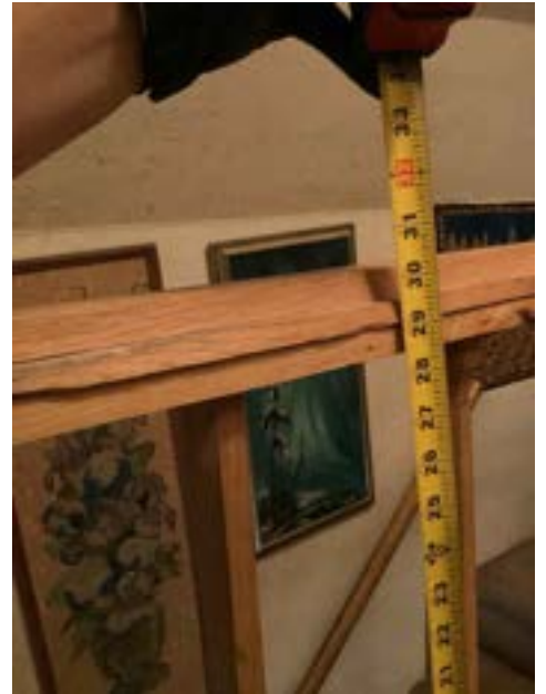
Insufficient Height of Guardrail - Hallway (Second Floor)
