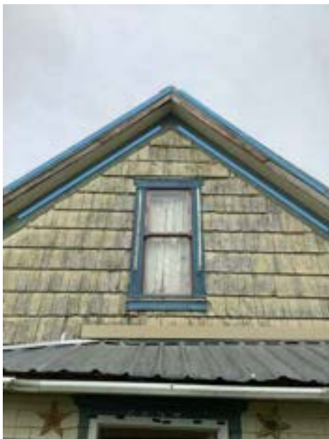
Fascia/Eave Paint Deteriorating (Representative Picture)
