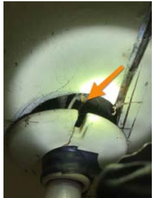
Junction Box Not Present - Side A
