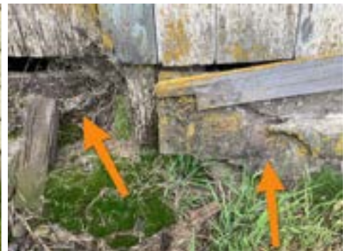
Skirting Wood Rot (Representative Picture)
