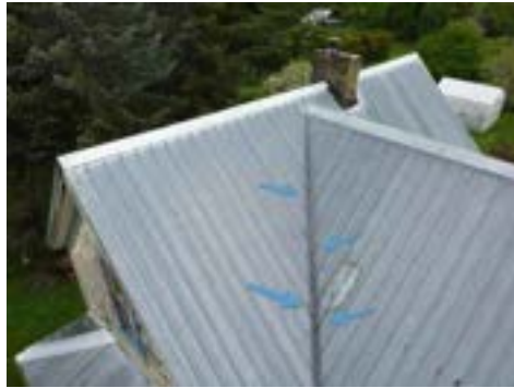
Corroded Roof Covering (Representative Picture)
