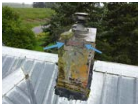
Chimney Mortar Deteriorating - Center Ridgeline
