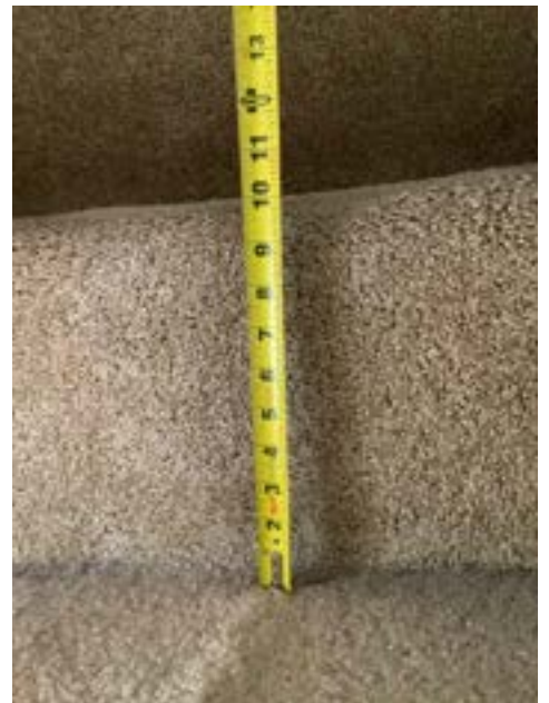
Step Riser(s) Exceed Recommended Height - Stairway (First Floor to Second Floor) (Representative Picture)
